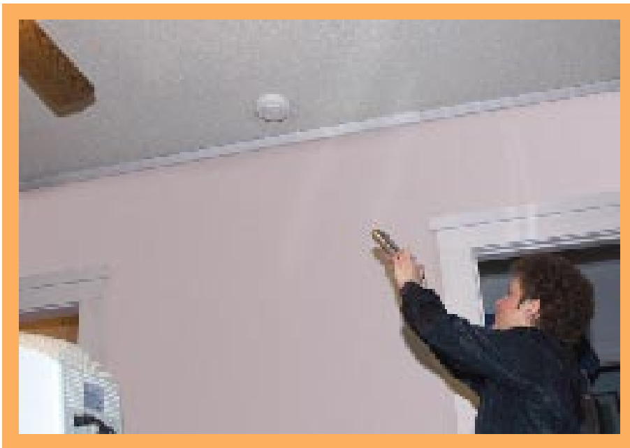
Figure 2: Point the remote toward the alarm.
